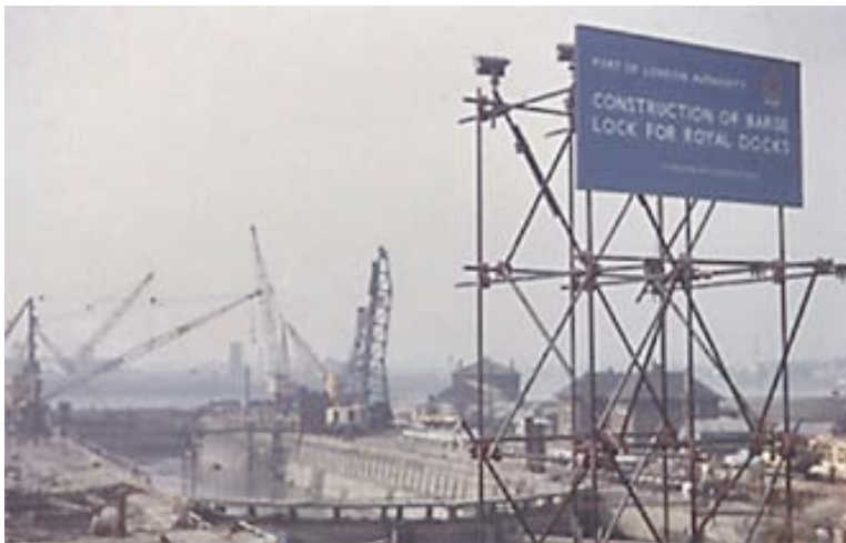
Figure 2: Work gets under way with heavy lift derricks and heavy piling rigs
